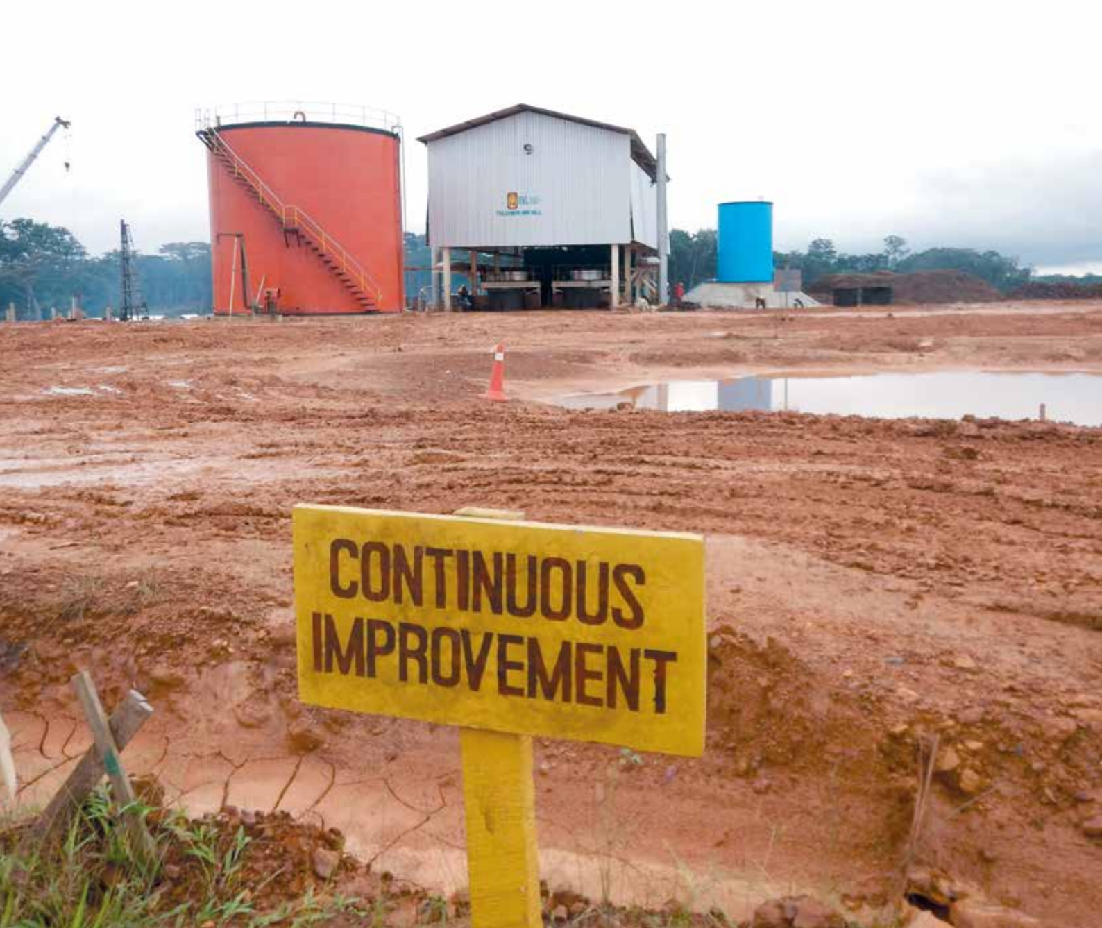
Company signboards at GVL construction site on Palotro Hill, June 2016. © Global Witness
